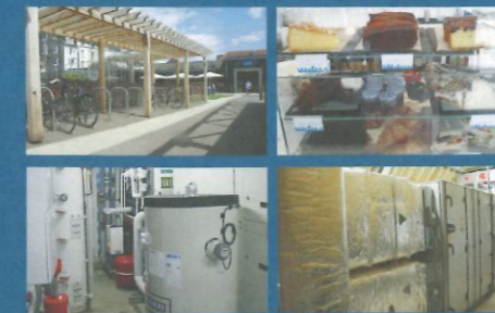
A parking lot for bicycles; the menu featuring locally sourced vegan dishes; Ground Source Heat Pump; air handling unit
